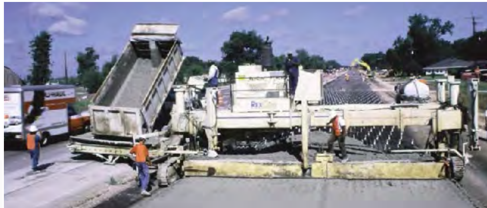
A number of highways in Louisiana were originally paved with CRCP. After a 25-year hiatus, the Louisiana DOTD used CRCP again, this time on US 190.
