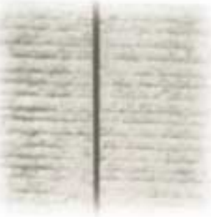
Longitudinal joint sawed at 12-foot centers to create highway lanes. Transverse rebar can serve as tie bars across longitudinal joints.
